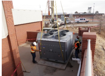
Chiller at Ft. Carson, CO
