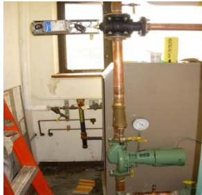
New Pumps, Valves APS Ops Bldg, Westover ARB, MA
