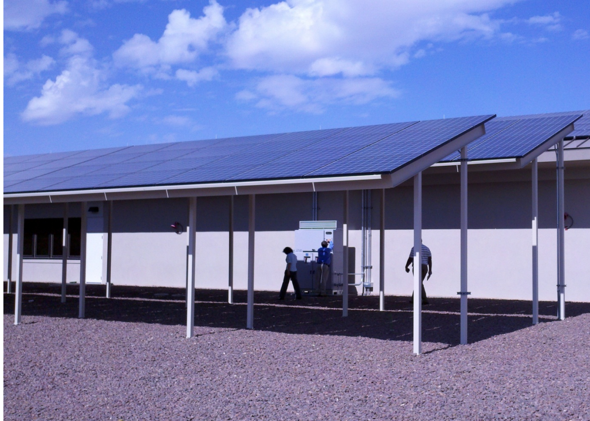
Ft Bliss PV Canopies
