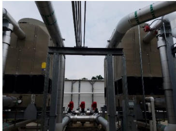
Cooling Towers at APG, MD
