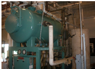
New Boiler at APG, MD
