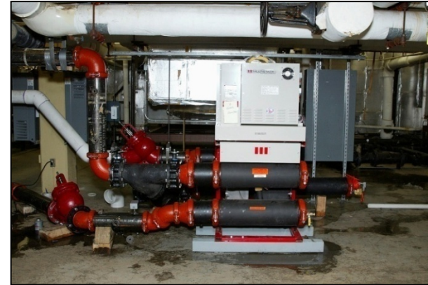
New Chiller with Magnetic Bearing Compressor at Newport
