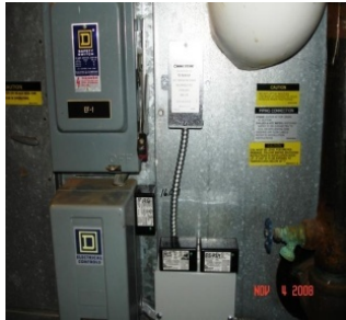
Relays and Controls, Sqd Ops Bldg, Westover ARB, MA
