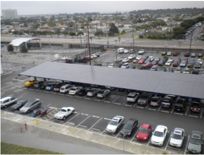
PV Parking Canopies LAAFB, CA & Ft. Bliss, TX
