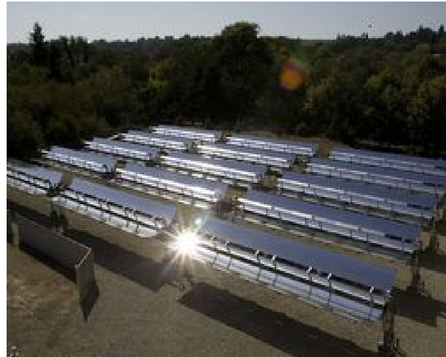
Sonoma Winery Solar Cogeneration Project
